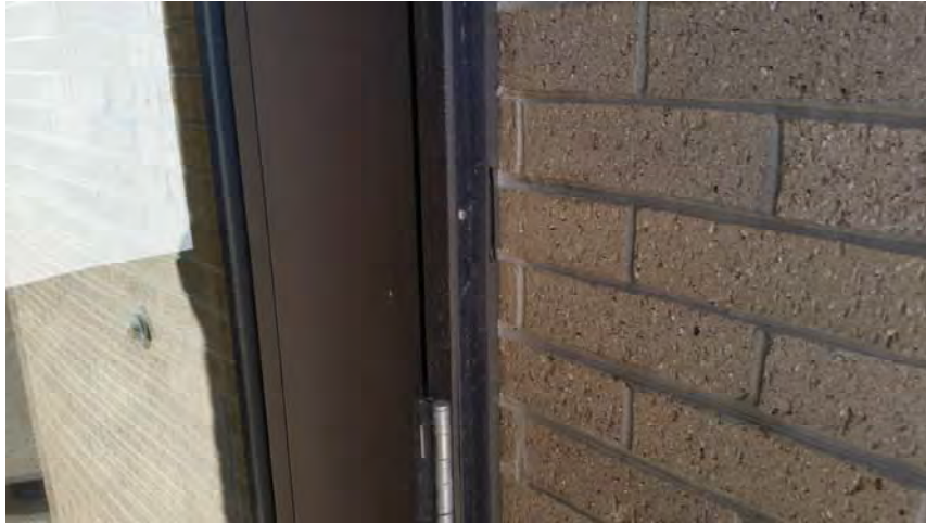
HA #31: Black Exterior Door Masonry Door Joint Sealant
