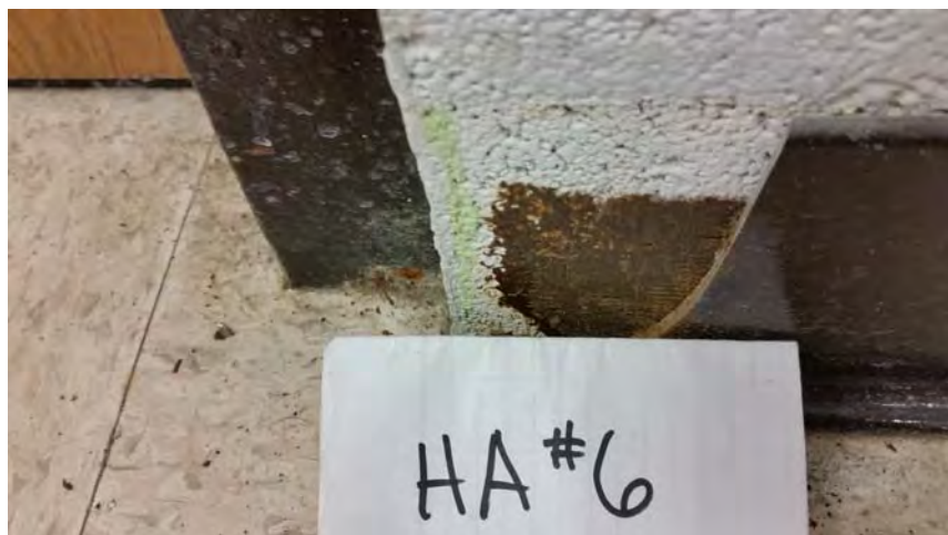
HA #6: Brown Vinyl Covebase Mastic
