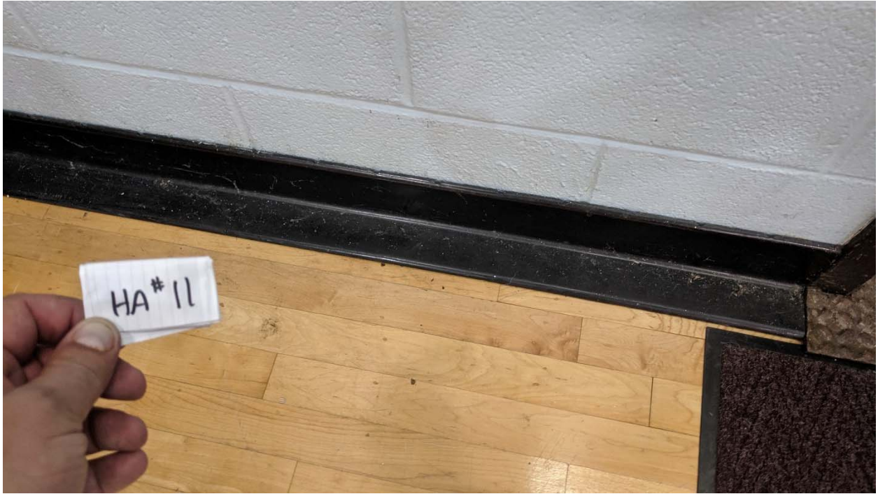
HA #11 – Black Vinyl Cove Base and Tan Mastic
