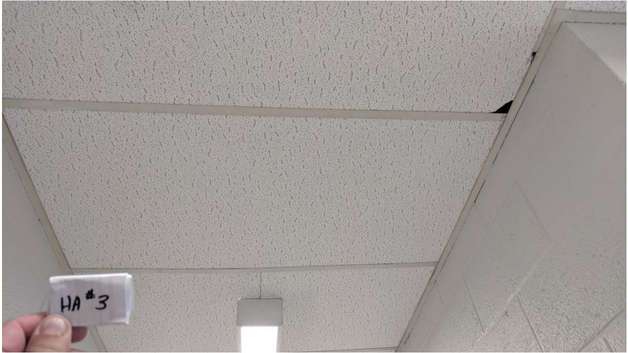
HA #3 – 2'x 4' White Pinhole and Fissure Acoustical Ceiling Tile
