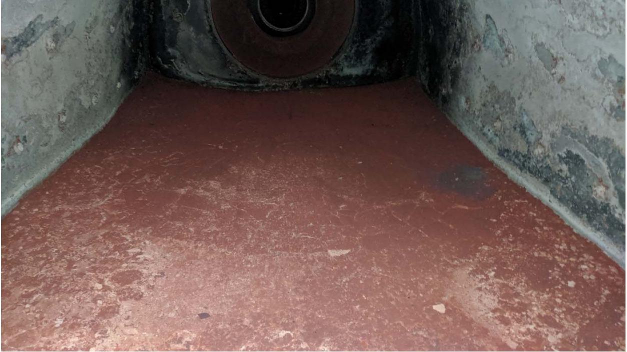
HA #26 – Red Lightweight Cementitious Boiler Liner
