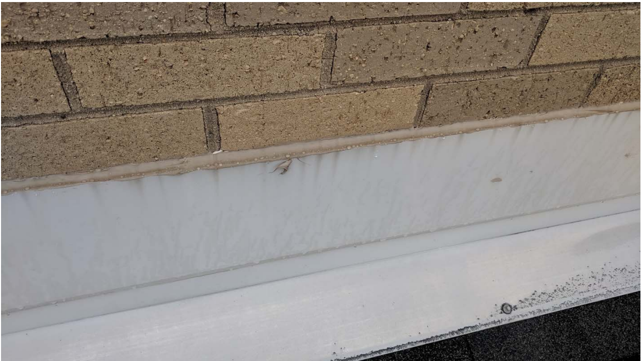
HA #23 – White Upper Flashing Sealant
